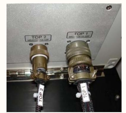
TO Panel Back showing TOP1 and TOP2 connected
