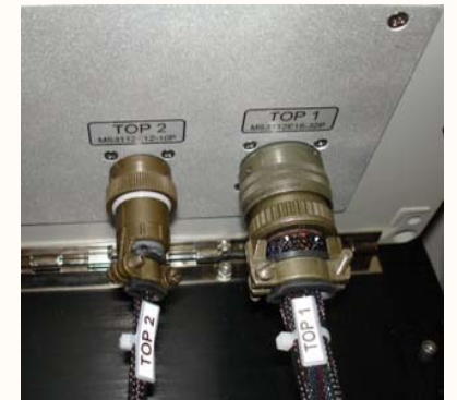
TO Panel Back showing TOP1 and TOP2 connected
