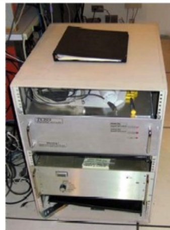
Facility Input/Output CD electronic box (top box) is currently located behind the TCS1 MCC equipment rack. The bottom box contains new power supplies for the TO area.
